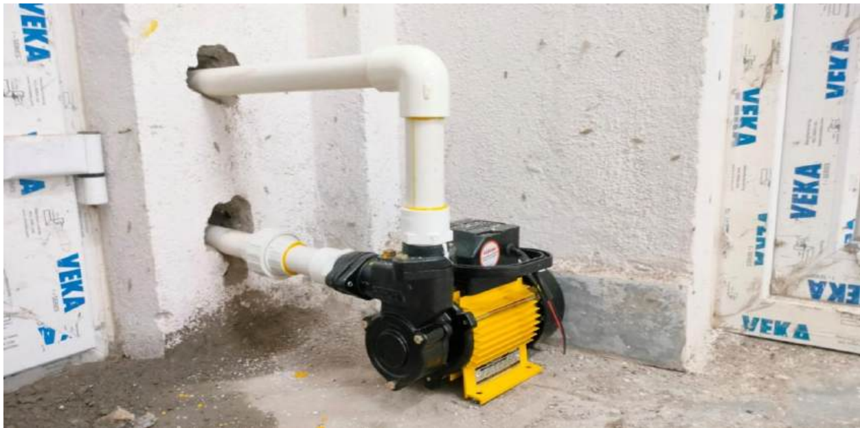
Water Pumping Motor
