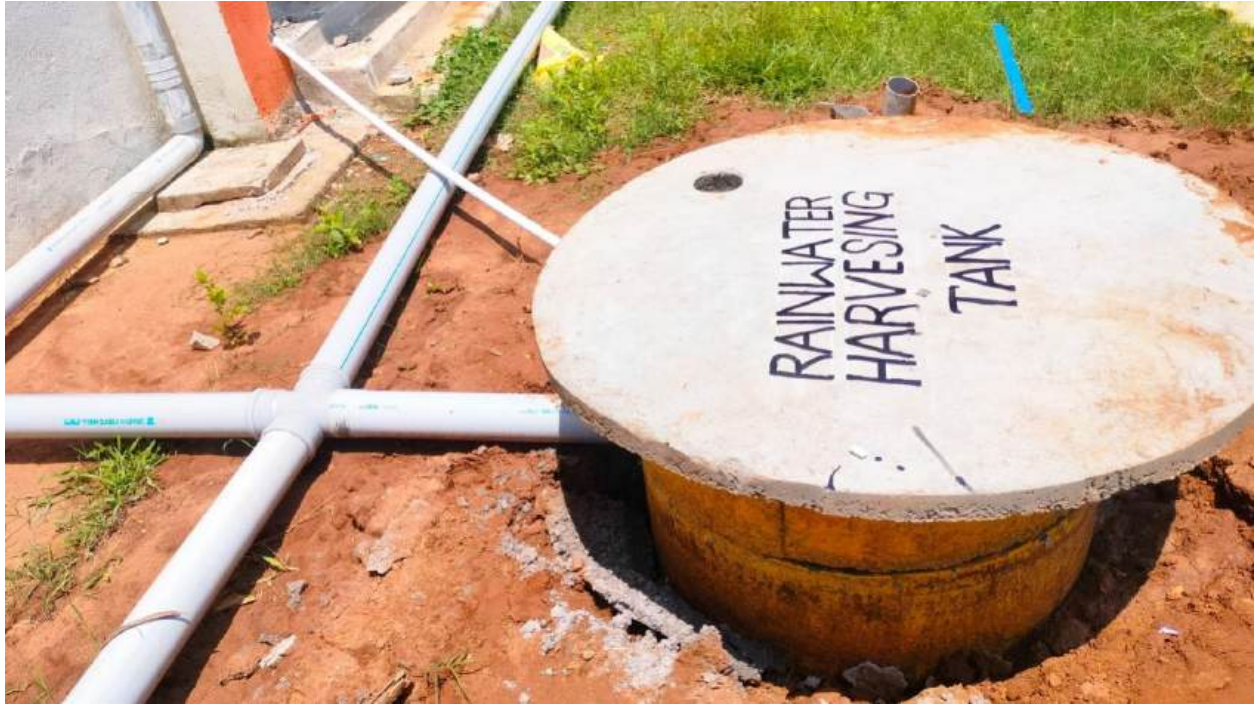
Rainwater Harvesting Tank (Storage Tank)
